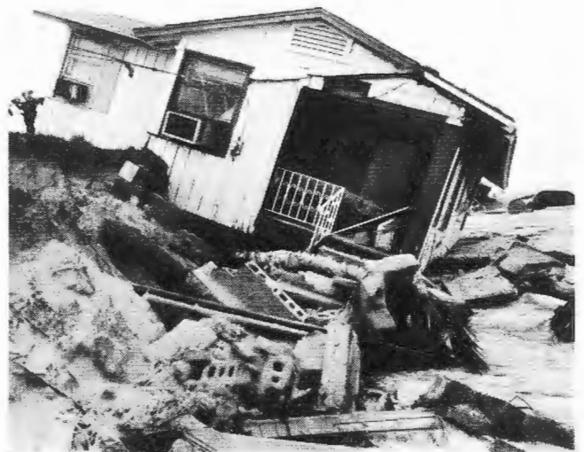
Figure 2.3. Erosion Caused This Foundation to Collapse.
